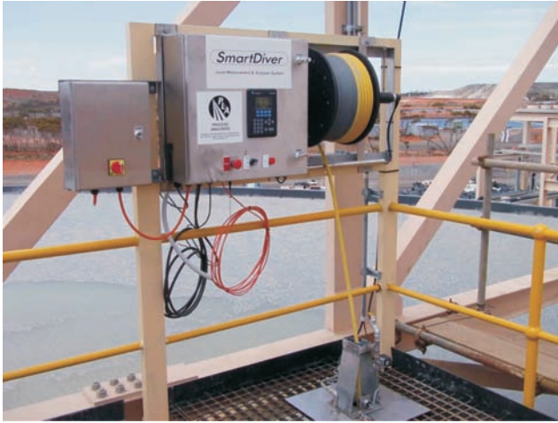
FIG 1 - A photograph of a Smart Diver installed at Gold Fields, St Ives.
